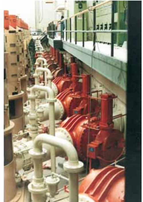
Ten 24" (600mm) Cone Valves Southern Nevada Water Supply
