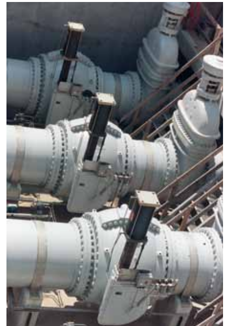
Coastal Water Authority, Houston, TX Lynchburg Pump Station Air/Oil Tandem Cylinders
