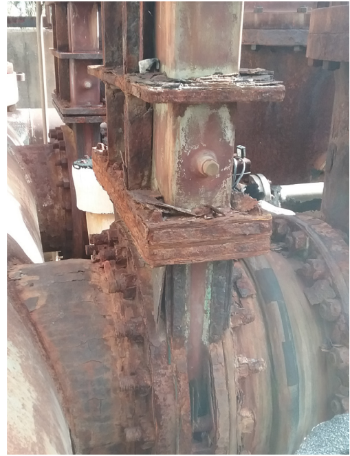
Knife gate valve with external carbon steel construction in a marine environment affected by MIC. Internal Monel wetted components were minimally affected.
