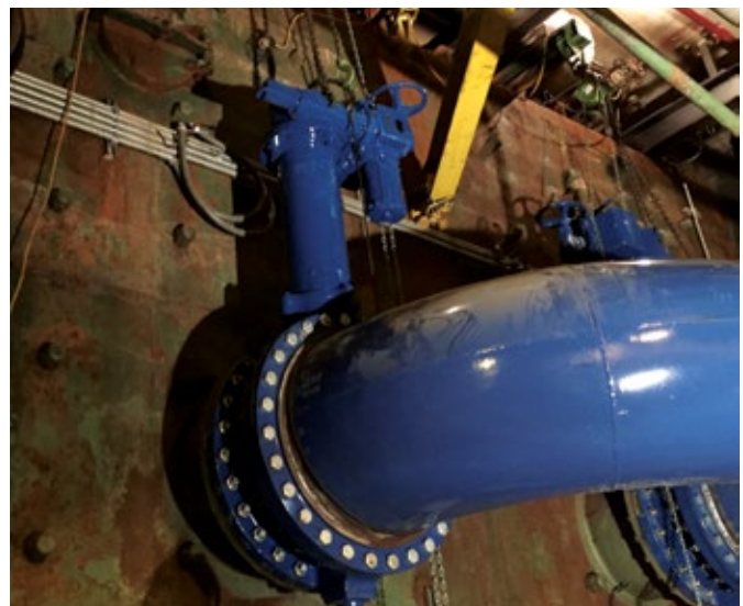
DeZURIK AWWA Butterfly Valves with neck extensions and electric motor actuators isolate water to the condenser.
