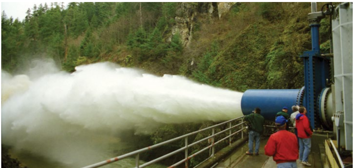
This 42" Hilton Jet Flow Gate is installed at LaGrande Dam near Tacoma, Washington.
