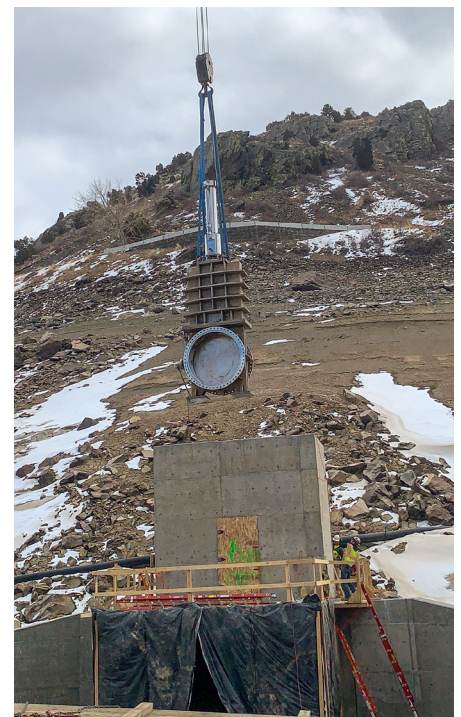
A crane lowers the 66" Hilton Knife Gate Valve down into the vault at the bottom of the reservoir.
