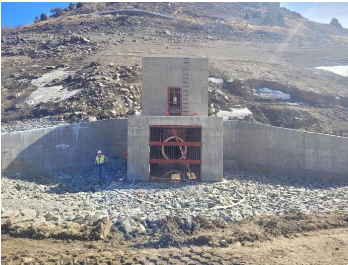
The 66" Hilton Knife Gate Valve in the vault at the bottom of the drained reservoir.
