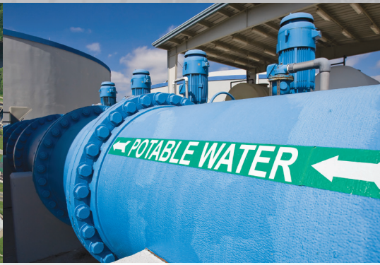
WATER TREATMENT & DISTRIBUTION
