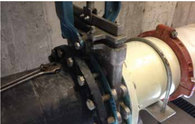
A DeZURIK Knife Gate Valve on a pond/ground water reclamation line.
