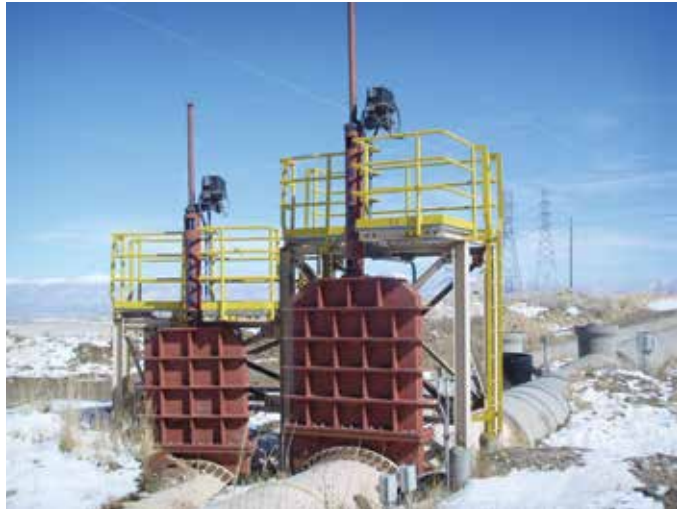
48" and 60" bonneted knife gate valves with motor actuators, carbon steel bodies, 304 stainless steel wetted parts and removable polyurethane port liners on a tailings application.
