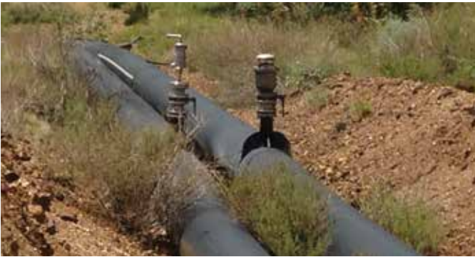
Slow Closing Air/Vacuum Valves on an acid delivery application.
