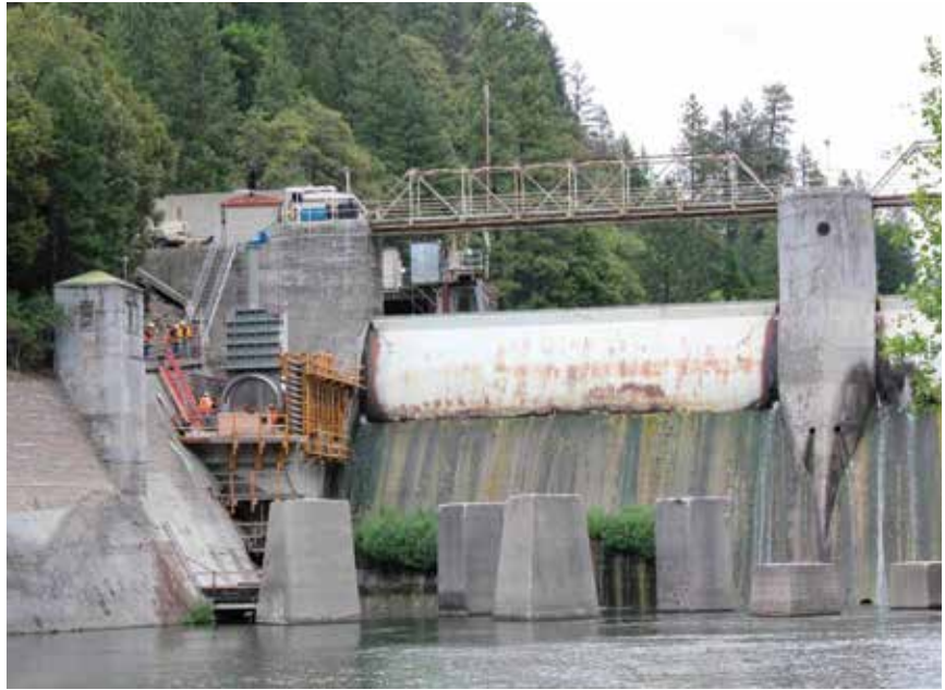
A 90"/102" Hilton Throttling Knife Gate Valve (30 psi rating) is installed on the Pit River in Northern California.
