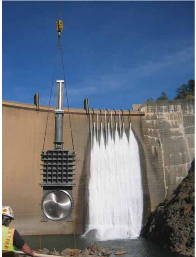
A 72" Hilton Bonneted Knife Gate Valve (130 psi rating) with 18" diameter hydraulic cylinder actuator is used for a guard valve for a fixed cone valve.
