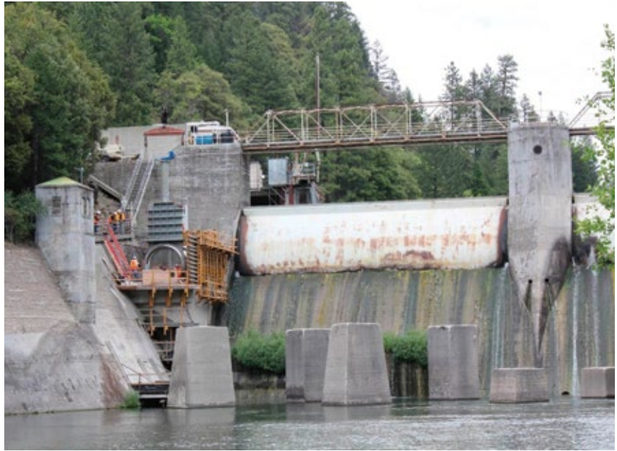
A 90"/102" Hilton Throttling Knife Gate Valve (30 psi rating) is installed on the Pit River in Northern California.
