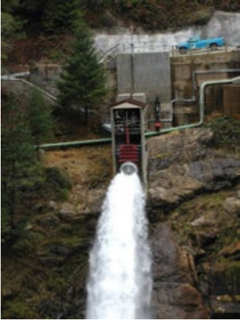
A 48"/60" Hilton Throttling Knife Gate Valve (50 psi rating) with electric motor operator is installed on a flow modification project.
