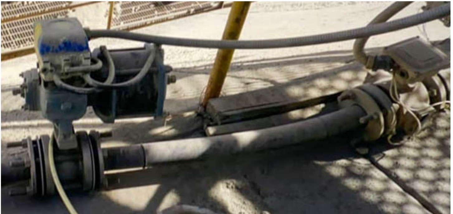
Raffinate Control - 2" RCV 317 stainless construction, full flow trim, PowerRac actuator, P201 positioner
