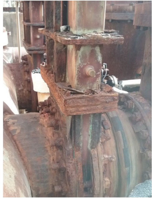
Knife gate valve with external carbon steel construction in a marine environment affected by MIC. Internal Monel wetted components were minimally affected.
